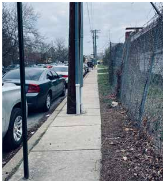
Narrow sidewalks on Reedbird Avenue have utility poles in the center, inadequate space for pedestrians to walk, and no landscaping or street trees
